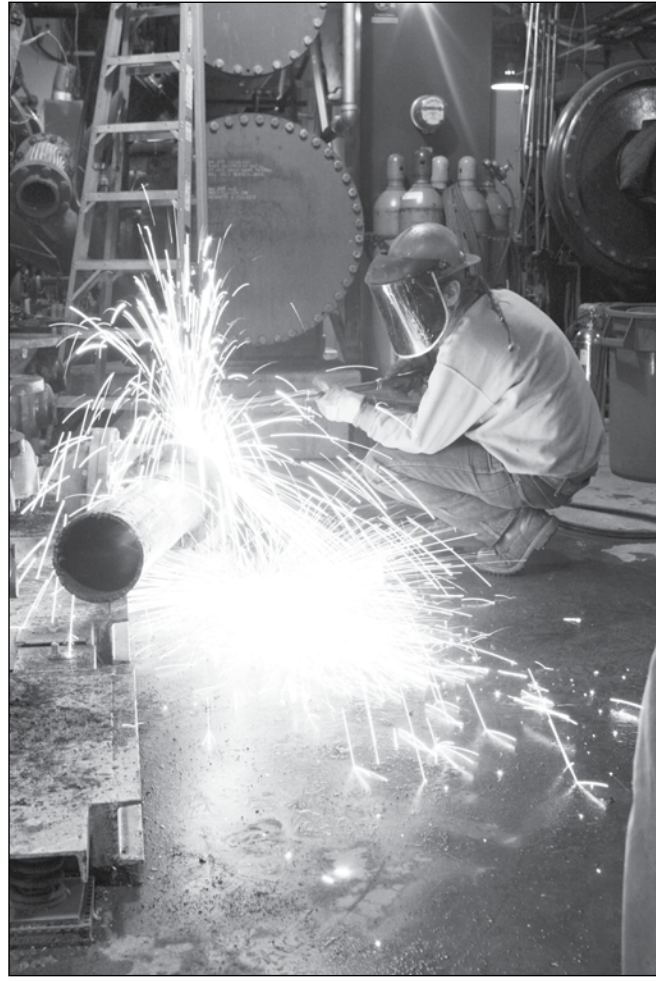
Photo by Brett Stanley/The Advocate Robert Terrill of Bockman and Sons Inc., a subcontractor in charge of demolishing the old air conditioning system, is working to remove the primary and secondary pump isolation valves.
